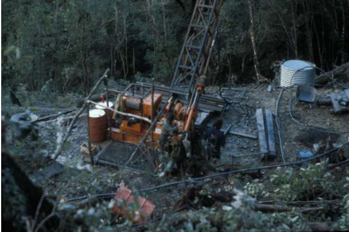
Figure 100 Drilling DDH MC1 at McConnochie Creek prospect by Gold Mines of NZ Ltd in 1980 (photo Franco Pirajno).
