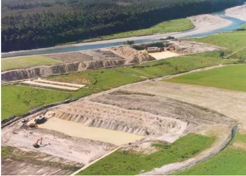
Figure 86 Restoration behind L&M Mining Ltd's No. 6 Plant (upper) and No. 2 Plant (lower) in the Arahura Valley. The No. 6 Plant is mining from left to right and the No. 2 Plant from right to left. Mined and restored ground is visible behind each plant. (Photo after Figure 5 of Manhire et al. 2006).
